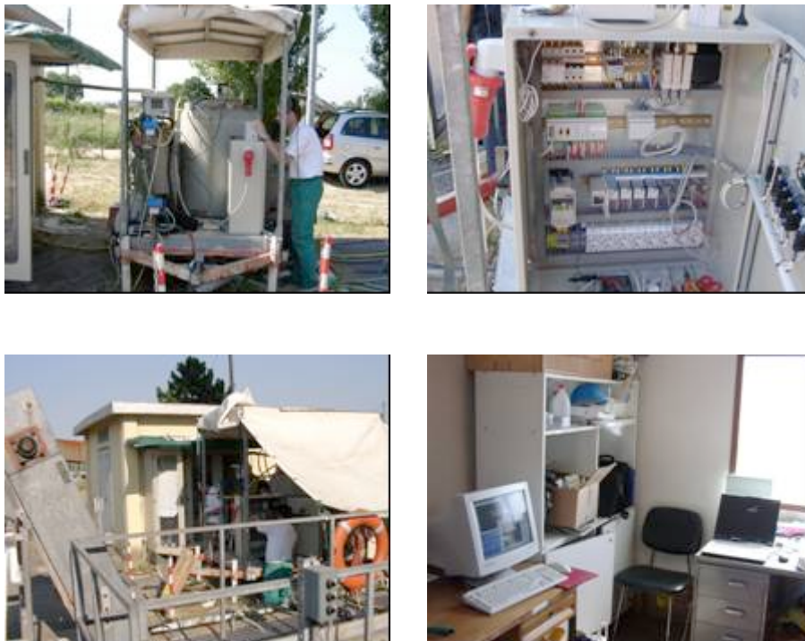
Figure 5: details of the electric cabinet set up and of the control room at the pilot plant in Bologna
