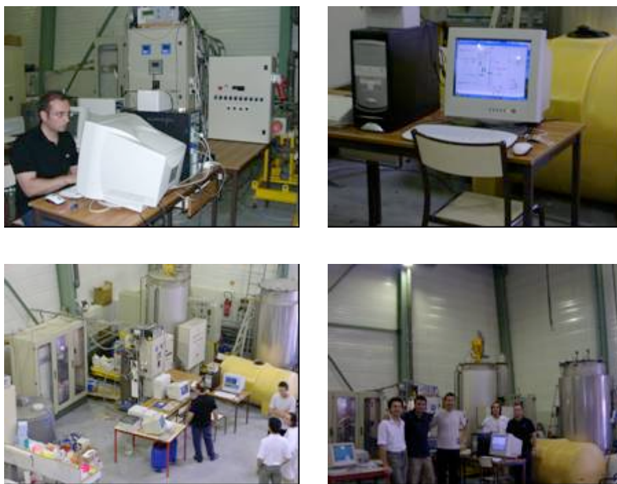
Figure 6: details of the electric cabinet and of the control workstation at the pilot plant in Narbonne
